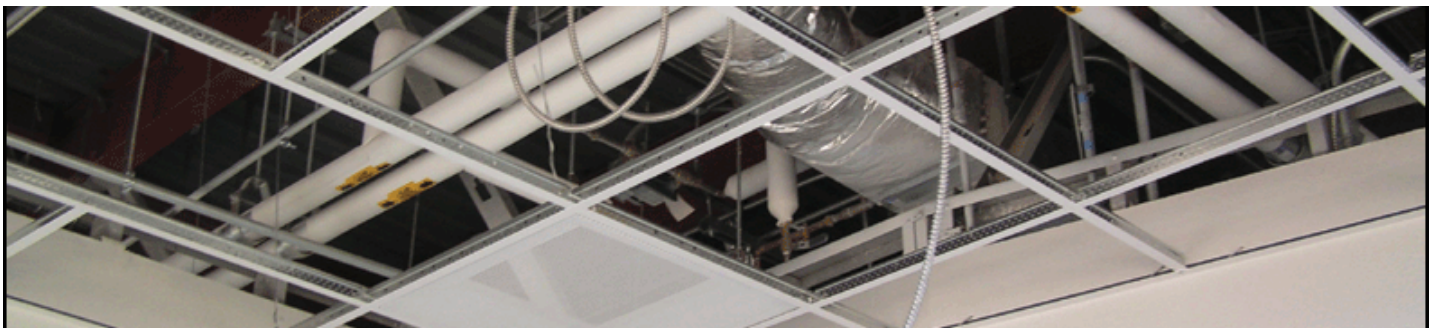
The ceiling grid is the single most important structural aspect of a modular cleanroom – make sure it remains true and level and that all components are functional, as well as properly seated and sealed. Photo courtesy of Technical Air Products.
